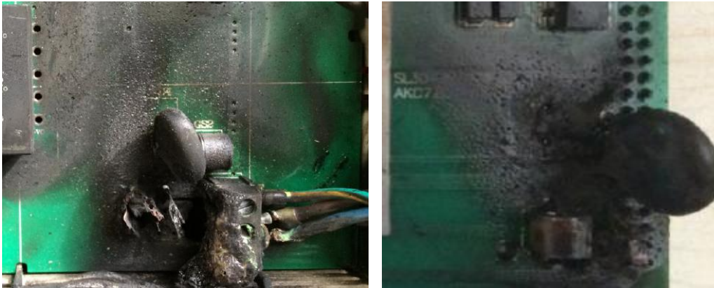
Figure 5. Burnt Circuit Board
